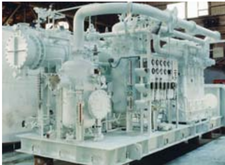
LPG Re-Liquefaction Plant (Nissin Gas Engineering Ltd.)
